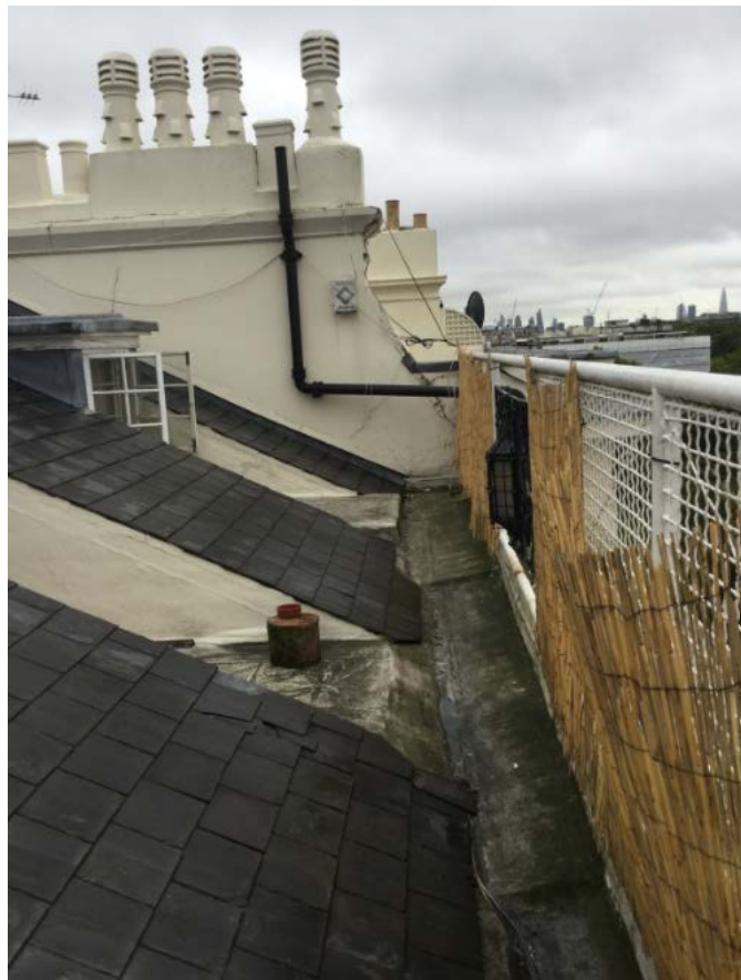
View of existing roof and dormers (top) and existing front roofslope and railings (bottom).
